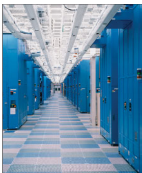
IBM is a worldwide leader in processor fabrication technologies, with a new $3 billion, state-of-the-art facility in East Fishkill, New York.
